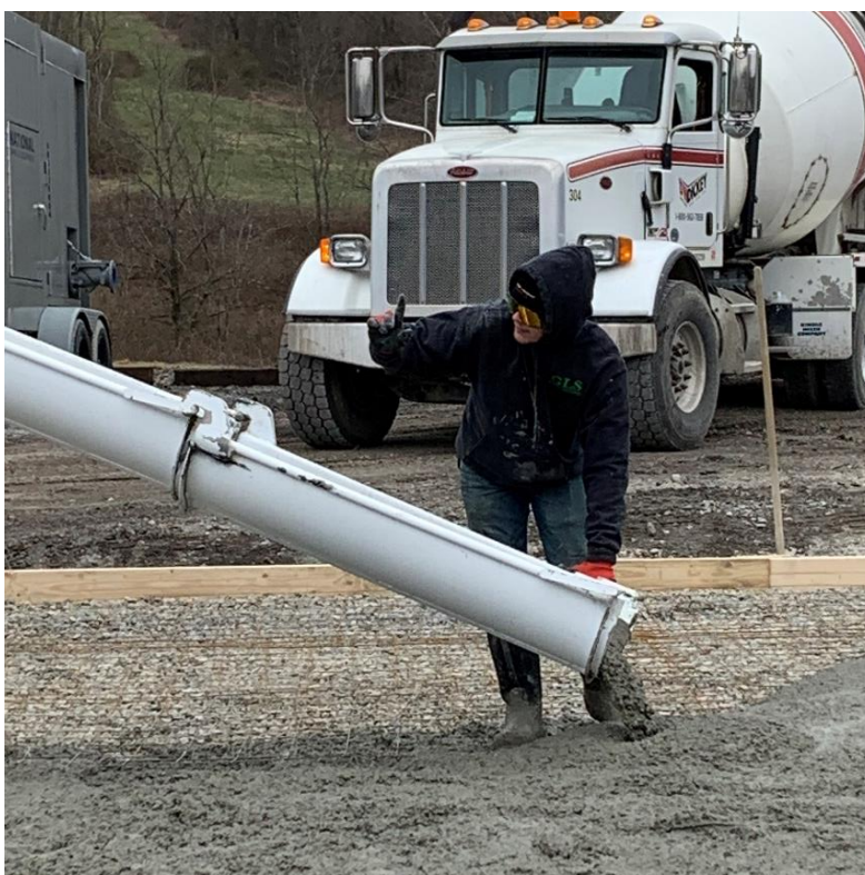
Cooperative Education student Mason Allison (B), employed by GLS Property Management, on the job pouring 80 yards of concrete.
